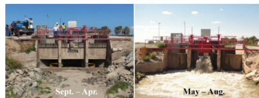
Figure 17. Installed units at Drop 8 Station
